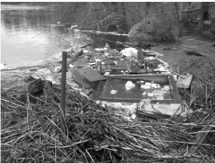
Sluce entrance of the Parke Memorial dam filled with debris immediately after the flood and before clean-up began. Photo by Duncan Schweitzer
